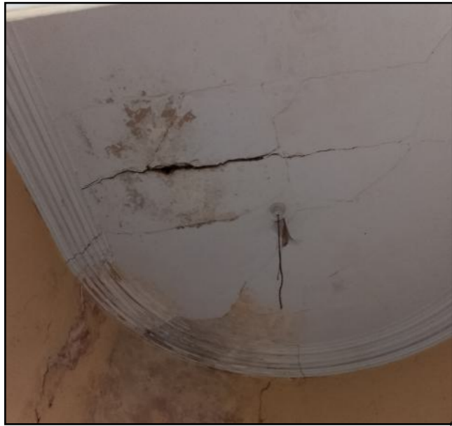
Cracks in ceiling
